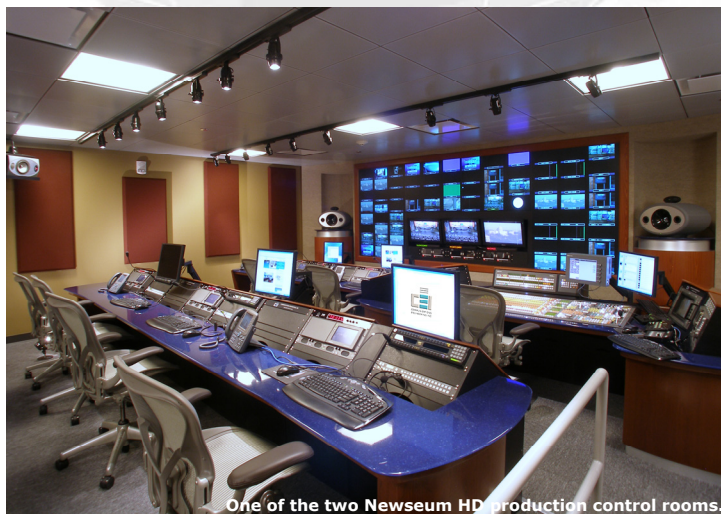
One of the two Newseum HD production control rooms.
